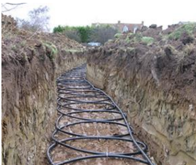
Photo left: Ground source heat pump pipework https://www.thermalearth.co.uk/agriculture
